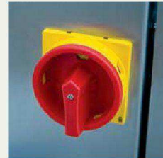
The main circuit breaker
